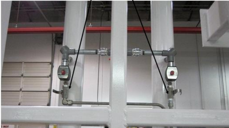
Isolation Valve at Point of Injection
