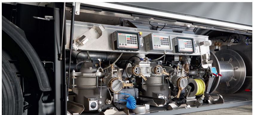
MultiFlow with dual GMVZ1004 meter gas extractor package in combination with NoMix (COP) on a service station delivery truck in Germany
